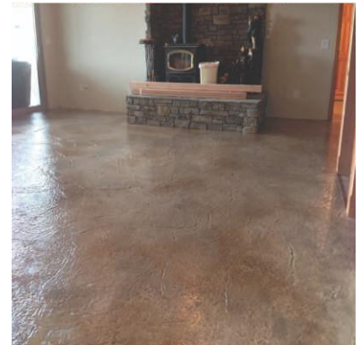
HICRETE STAMPED OVERLAY FLOORING
